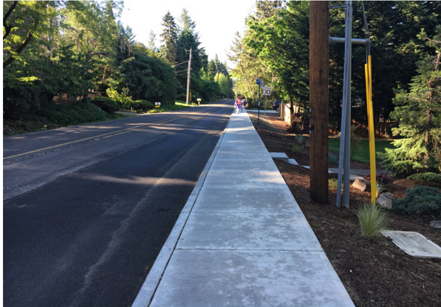
A stretch of sidewalk on Southwest 90th Avenue, from Southwest Washington Street to Southwest Morrison Street, is one project being tackled to improve safety in unincorporated Washington County. (Courtesy of 3j Consulting Inc.)
